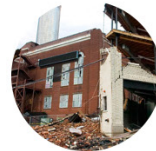
A tornado in 2008 destroyed part of the lofts and many historic homes. The community came together to recover the neighbourhood
